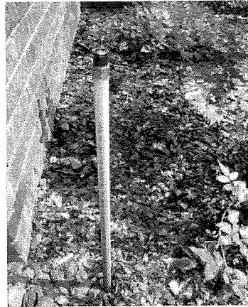
Figure 5. Shrubs adapter and fixed nozzle on riser
