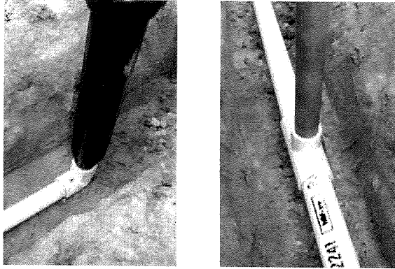
Figure 128. Incorrect sprinkler connections
